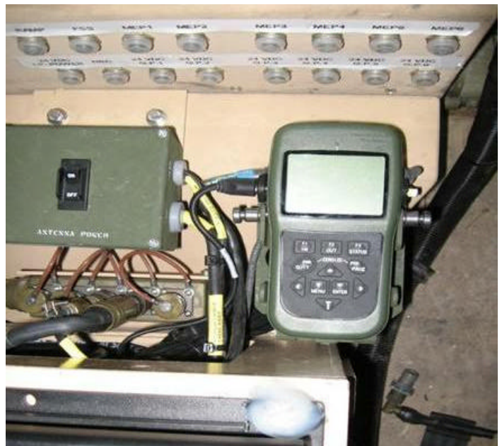
The improved installation of the DAGR as seen from approximately the same camera angle as shown at left but now the DAGR is seated against the center console in the same orientation as the antenna switch box. The 90 degree antenna cable on right side presents a smaller target for unintentional contact and the power cable on the left side is better protected as well.
