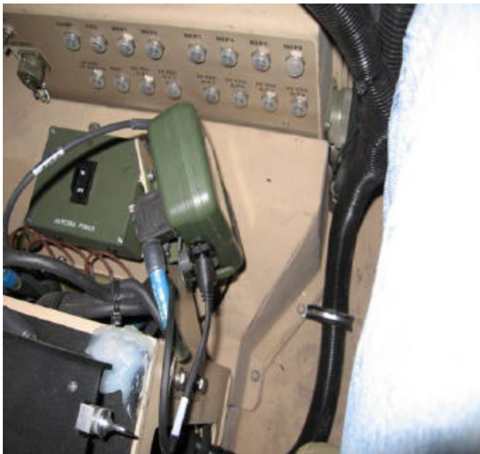
The initial DAGR installation as seen from vehicle commanders view, looking down at center console. Note the remote power cable extending alongside the seat edge which makes it prone to being snagged as crew enters or exits the front seat. This location also requires the crew to lean forward and twist to see the DAGR display! Also note the remote antenna cable at top of DAGR hangs over the master antenna switch (green box).
